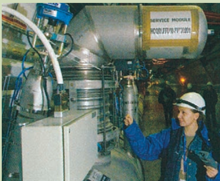
The first section of the cryogenic distribution line, corresponding to an eighth of the accelerator, has been tested at a temperature of 10 K since the end of November 2005.
